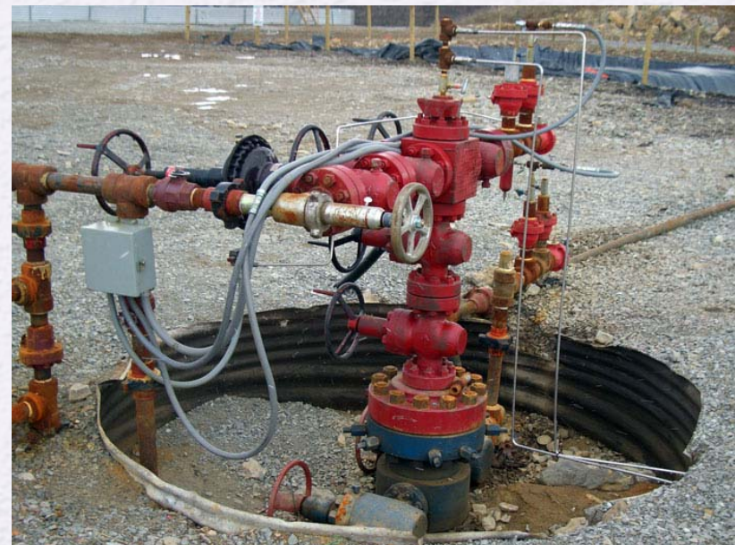
Wellhead, Hickory, PA. http://www.donnan.com/images/Marcellus-37.jpg
