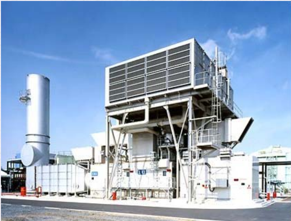
Natural Gas Power Plant in Russia
