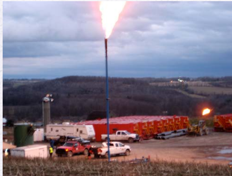
Well pad with storage tankers and flares burning
