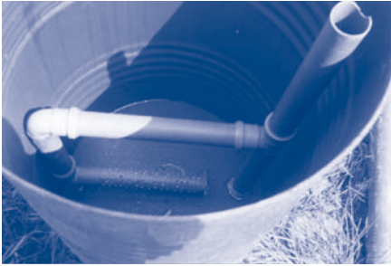
Pipe arrangement for sand filter
