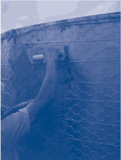
Application of the first layer of mortar on top of the wiring
