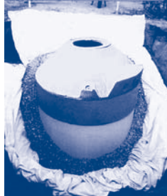
A precast concrete tank being buried in urban Germany (Picture: Mall GmbH)
