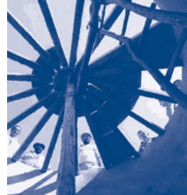
Precast plates being placed on a ferrocement tank in Brazil (Picture: Johann Gnadlinger)
