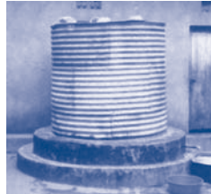
A corrugated steel tank in rural Uganda. Note the darker ring at the bottom of the tank – a concrete repair that is often needed (Picture: D. Rees)
