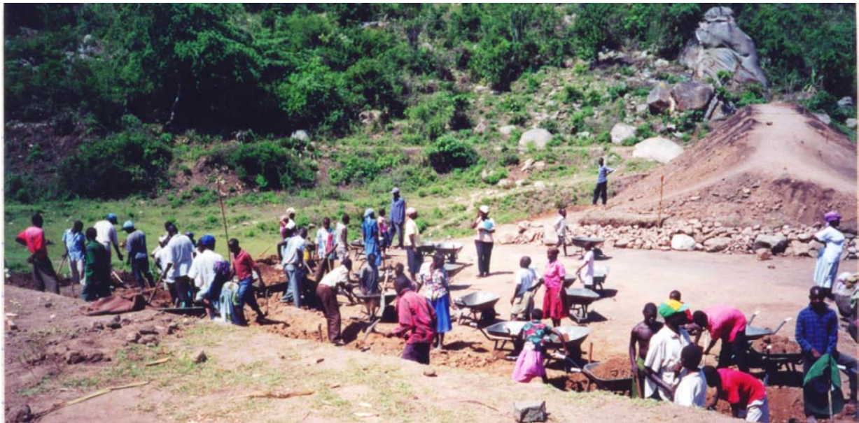
A spillway is being excavated for the manual construction of a valley dam with a straight embankment in a narrow part of a valley near Lake Victoria in Western Kenya.
