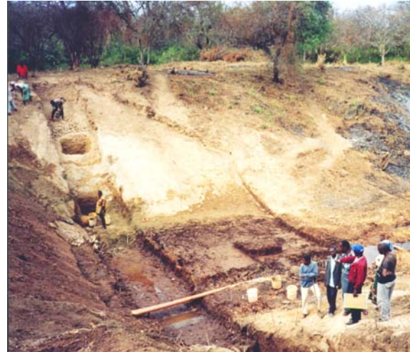
The key has been excavated into solid soil with some test pits to prove that there are no layers of sand underneath the key.
