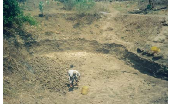
Unfortunately, this farmer has only one shovel and 3 old jerrycans to excavate and transport soil.
