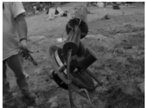
Figure 36 - Slide the wires through the tower top, while a helper lifts the wind turbine into place on the tower stub.
