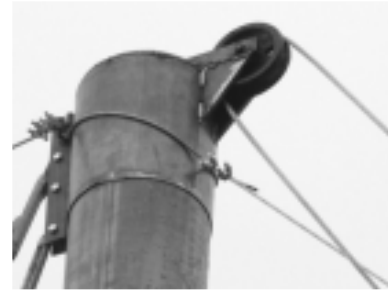
Figure 29 - Pulley at the end of the gin pole, to give a mechanical advantage while raising and lowering.
