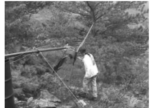
Figure 26 - Maintaining a wind turbine while standing safely on the ground. We love tilt-up towers for this reason!
