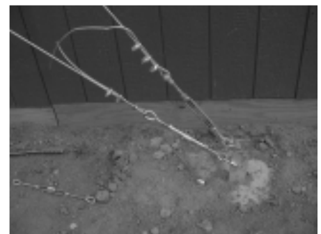
Figure 33 - Guy wire anchor embedded in concrete.
